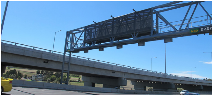
T100/T200 Level Sensors on Melbourne's M80 Ring Road
